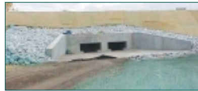
Photo: The storage basin's inlet/outlet structure is located at the deepest point and serves to fill and dewater the basin.
